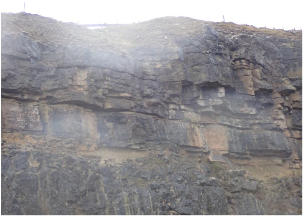
Plate 30: upper rock section with rockfall debris on ledge of weaker materials (recent rockfall).
