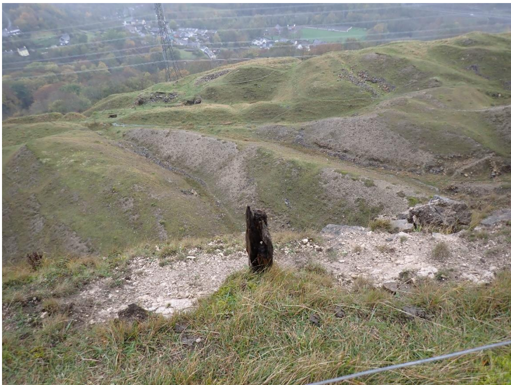
Plate 16: Chainage 135m, slip on slope below road close to carriageway.
