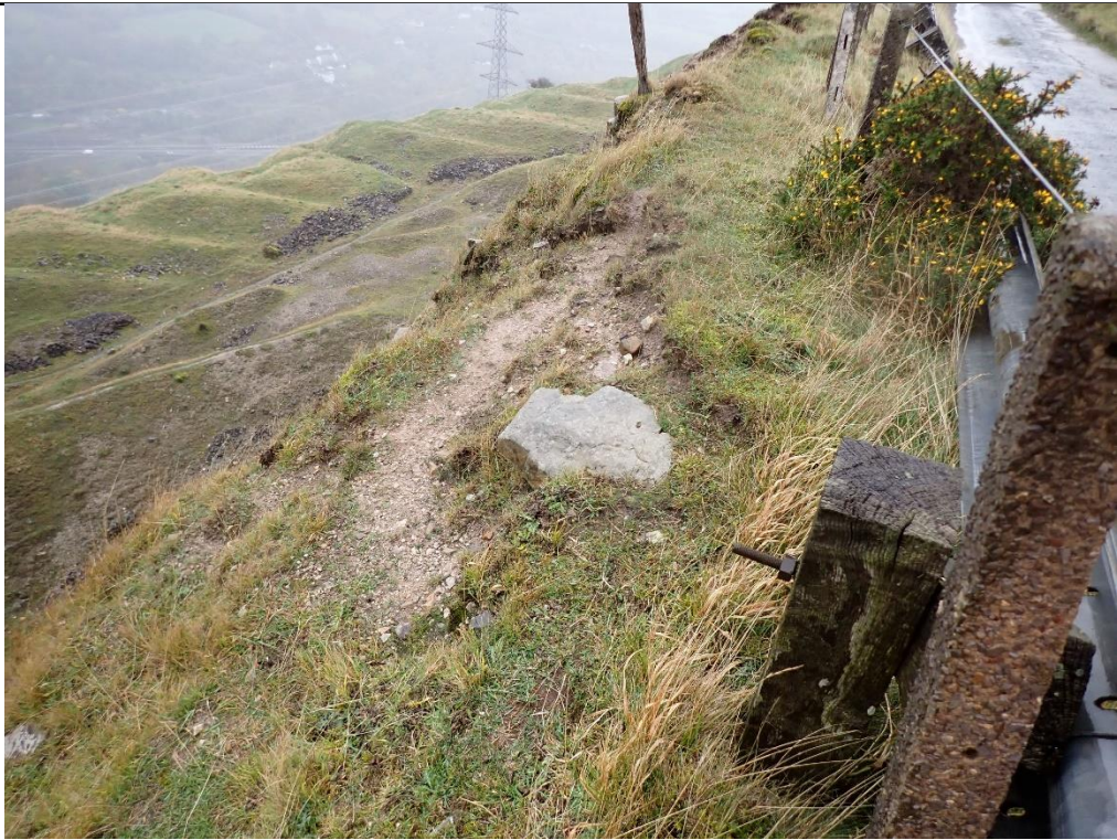
Plate 19: Chainage 150m, slip on slope 1.5m off highway
