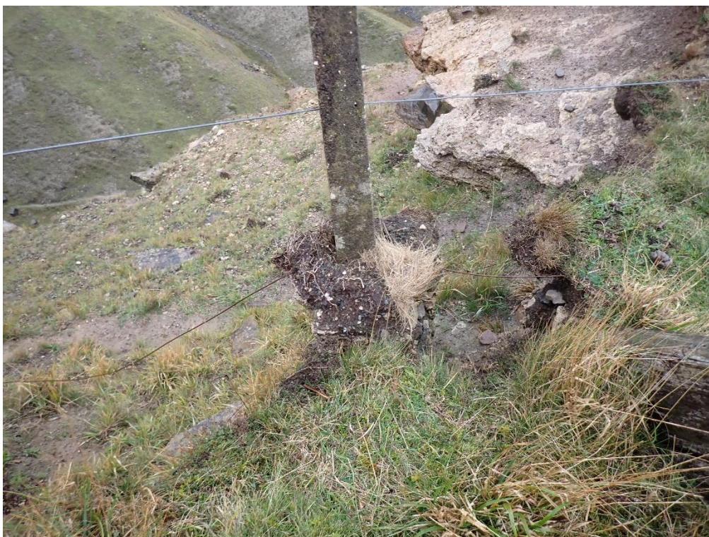
Plate 14: Chainage 100, failed fence post foundation.
