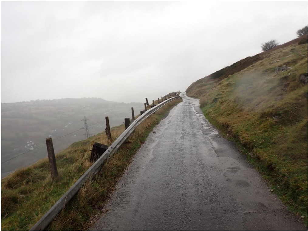
Plate 15: Chainage 104 to 112m, failed tilting VRS.
