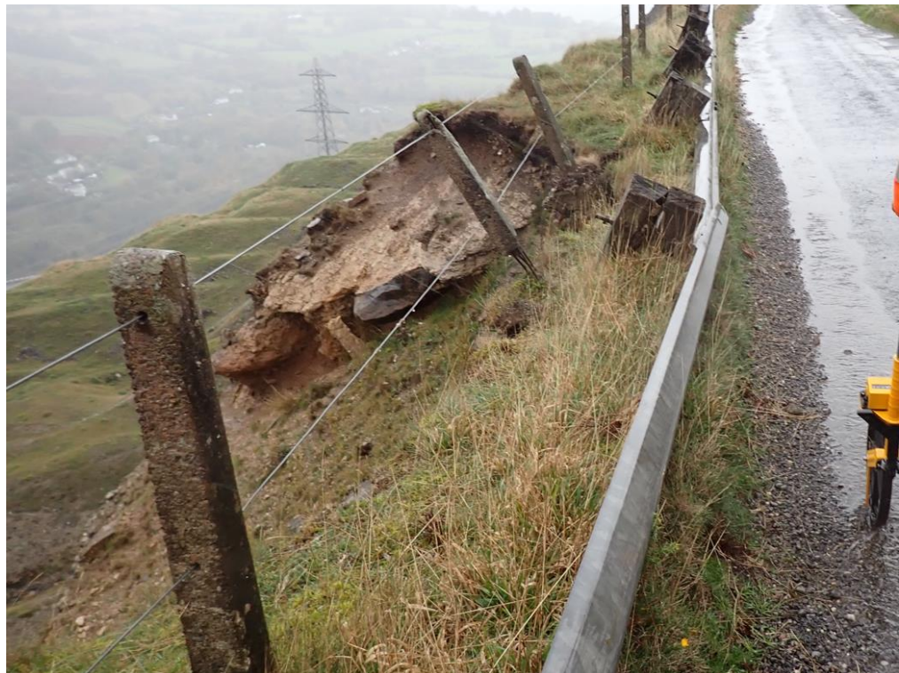
Plate 12: Chainage 97.0m to 112.0m, crest of slope close to road edge, slip in slope below, rotated VRS and fence post.
