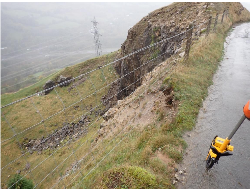
Plate 26: Chainage 243, Section of fence with no support due to crest failure with grip through verge.
