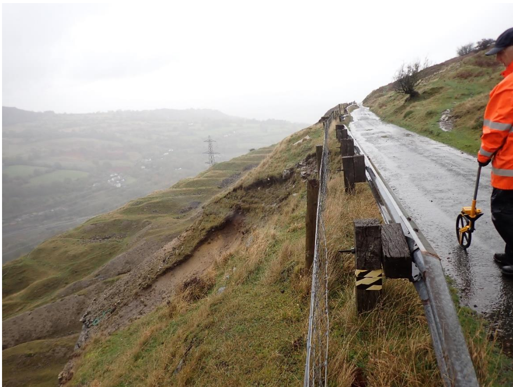
Plate 6: Chainage 69m The rock face / crest of slope moves within 0.5m of the back of the VRS
