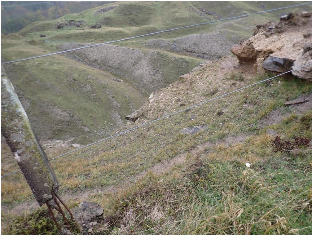
Plate 13: Chainage 97m, slip bowl below the road above quarry face with unsupported post
